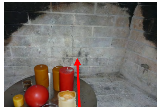
Cracking noted at firebrick
