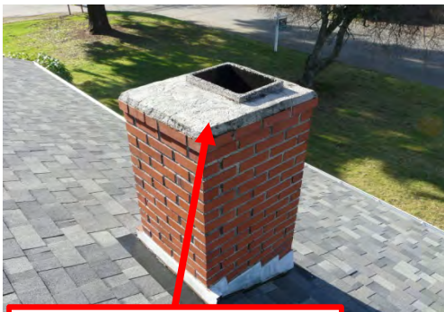
Spark/rain caps absent at chimneys.
