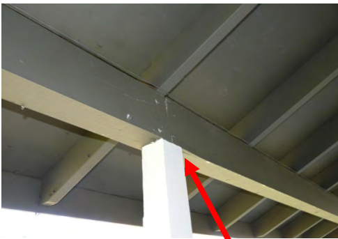
Front posts not mechanically connected to beam.
