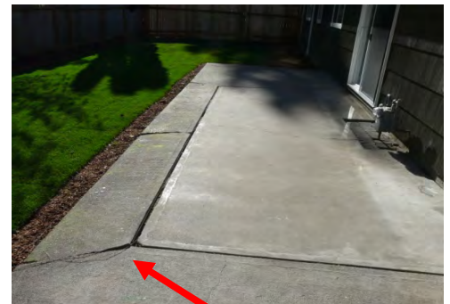
Settling noted at parts of the back patio.
