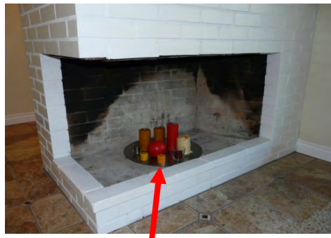
No screen or glass in place at main floor fireplace.
